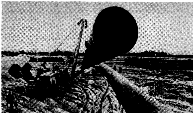
Pipeline construction in Siberia could soon provide West Germany with a large part of its natural gas needs.
