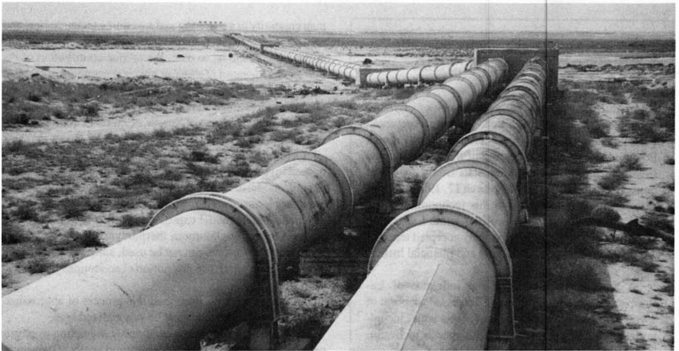
This pipeline, built during the Soviet period, brings water from the Caspian Sea to a desalination facility in Shevchenko, Kazakhstan. A Eurasian development program must build infrastructure in the vast, undeveloped spaces east of Warsaw.
