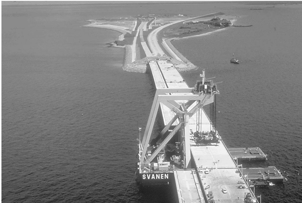
A view of construction on the West Bridge section of the Great Belt Fixed Link project. Most often, the concept of new technologies is associated with computer science, space programs, or other exotic technologies. But an often-overlooked aspect of large-scale infrastructure projects, is the development of new technologies.
