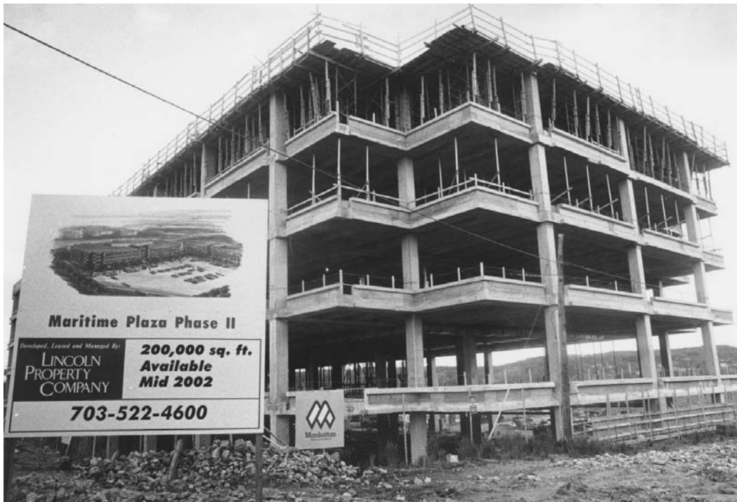
Office building construction in Southeast D.C., in the triangular area just east of the Navy Yard; according to the Washington Business Journal, it is hoped that this project, along with others, “could help build the momentum for a major transformation of this historically underdeveloped area.”
