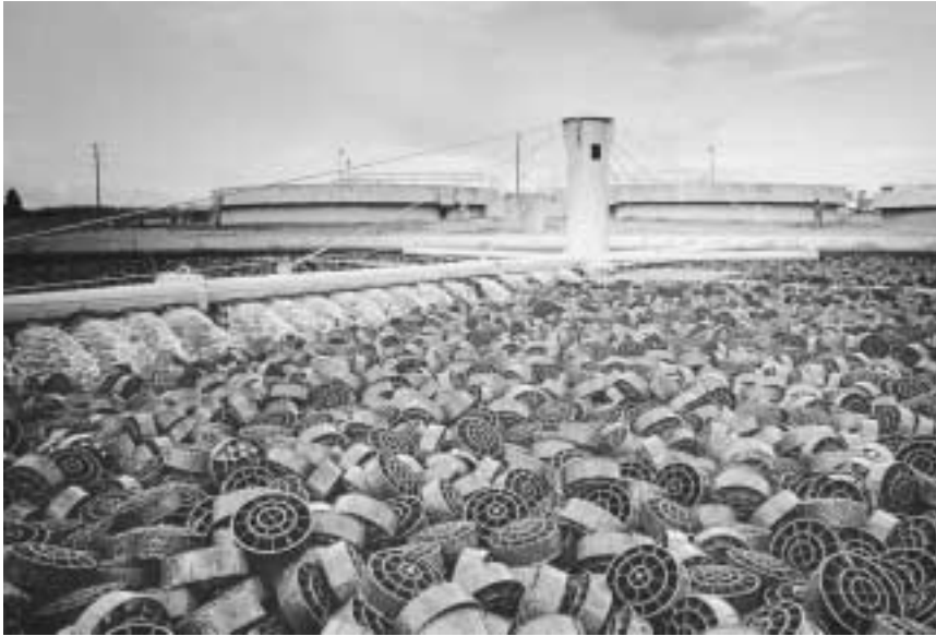
Filtering media of a 15-year-old sewage treatment plant in Virginia. Vast amounts of U.S. water treatment and runoff infrastructure is four to ten times that age, and breaking down; our national water-treatment “debt” is near $1 trillion in replacement costs.
