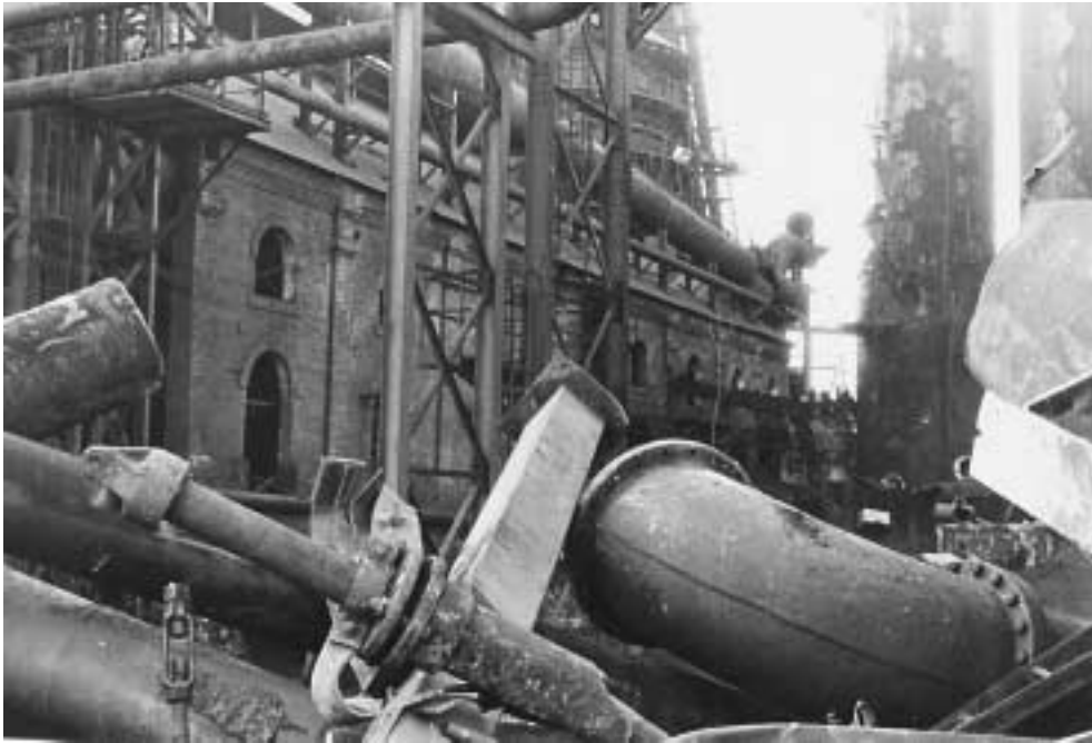
Demolition of a steel mill in McKeesport, Pennsylvania, in 1985. American populists cut their own throats by supporting free trade and deregulation, in the interest of getting a “cheaper deal.” The result: no U.S. economy!
