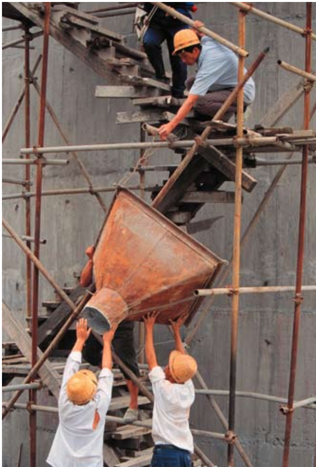
Workers constructing China's Three Gorges Dam, now the largest source of hydroelectric power in the world. The dam is a useful project, but it's not enough for a country the size of China.
