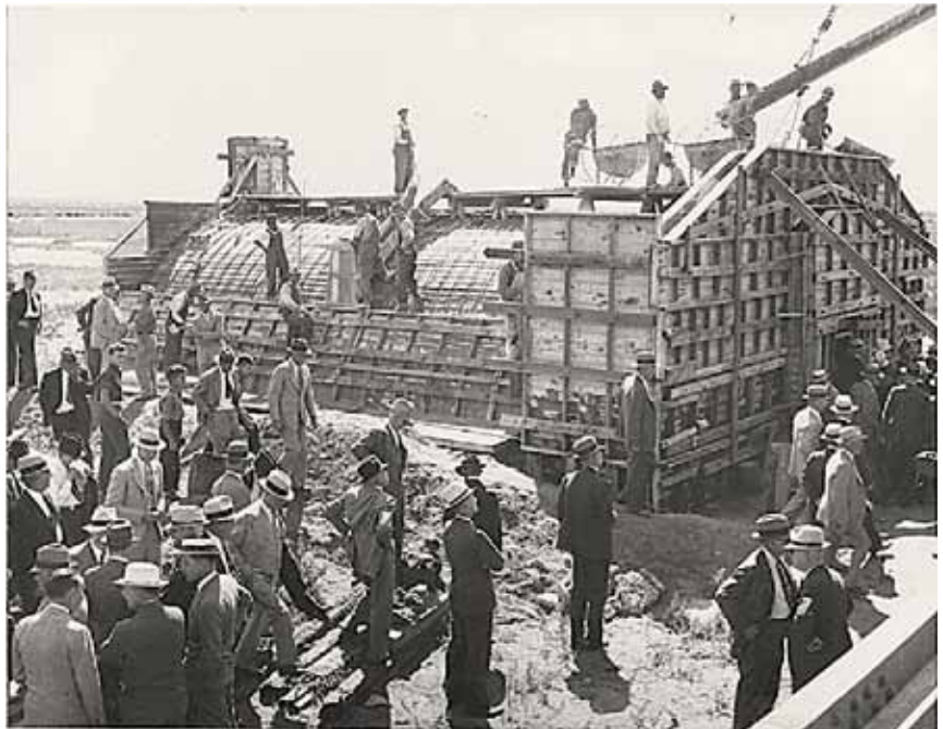
The WPA (Works Progress Administration) was a “school,” “a parking place to keep people alive economically, until we could get them employed in real skills.” Here WPA workers pour concrete on a storage unit in Ogden, Utah, in 1936.
