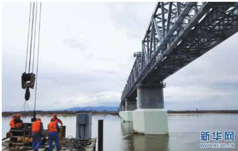
Railroad bridge nears completion, linking Tongjiang City in northeast China’s Heilongjiang Province with Nizhneleninskoye in Russia’s Jewish Autonomous Oblast.
